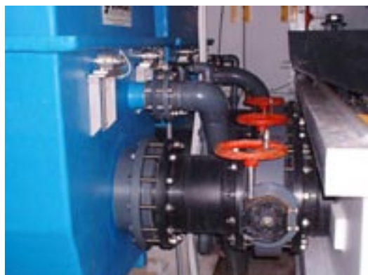
Three filters HDF1203-1P installed in parallel. Inlet valves to each filter.
