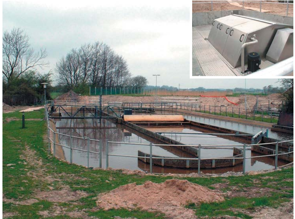
Main picture: Oxidation ditch, modified A-channel
